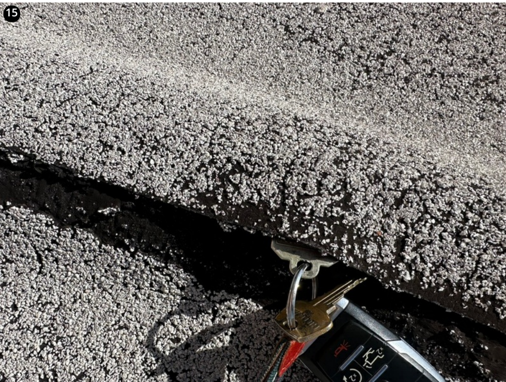
Open seam on a blister along--typical throughout.
