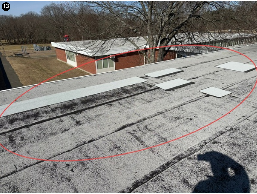
Patches throughout from previous blister repairs
