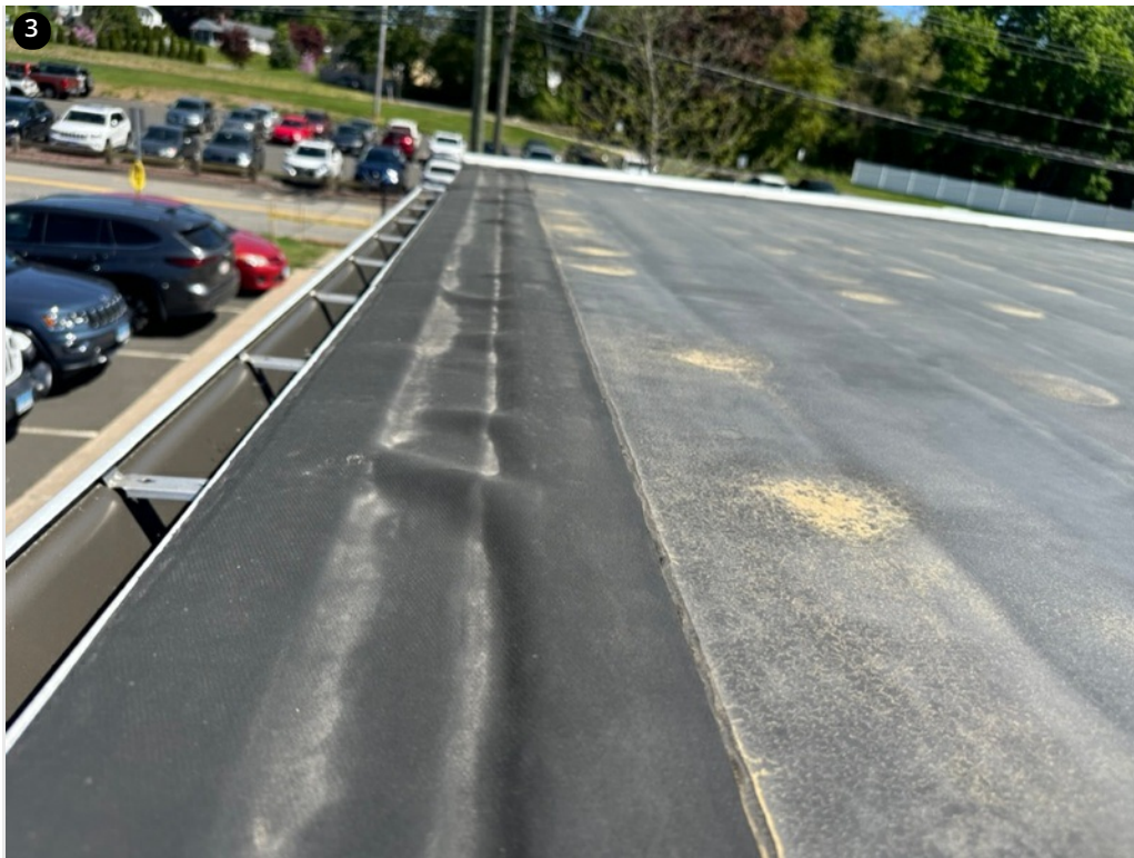
3 Perimeter of this section-- perimeter cover strip is starting to delaminate.
