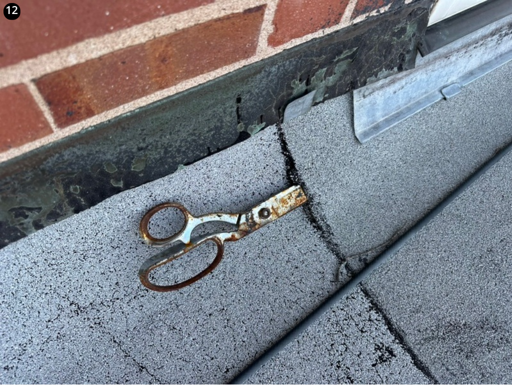
Large open condition at a flashing seam-- typical
