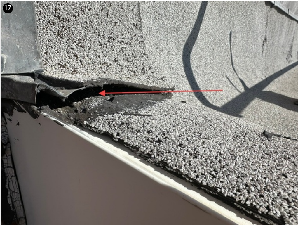
Failed flashing seam and large open condition--typical.
