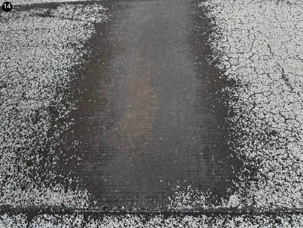
Close view of the mineral loss- this is pretty severe and prevalent throughout in varying severity
