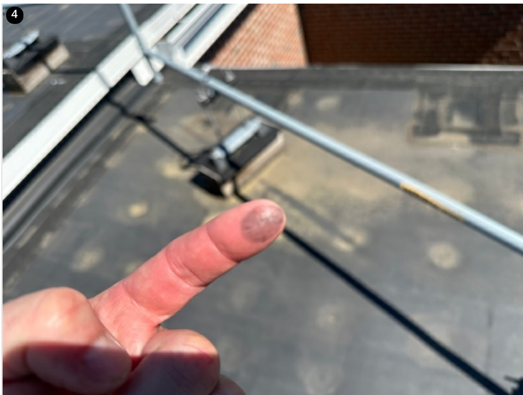
4 The chalky/gray color and staining is a typical sign of aging. As rubber is exposed to UV, the chemical compounds evaporate. As this progresses, over time, the water proofing slowly diminishes until it the roof fails.
