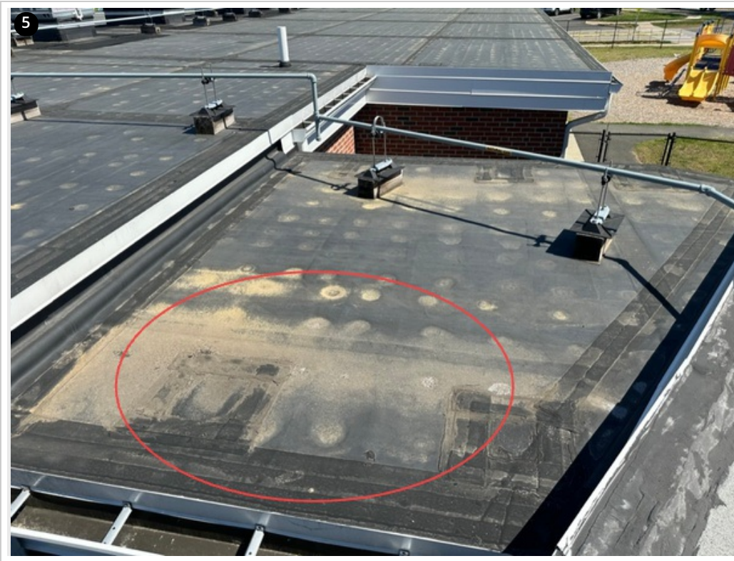
Debris build-up on the roof, indicating a lack of proper pitch and ability to drain water to the drains/gutters.
