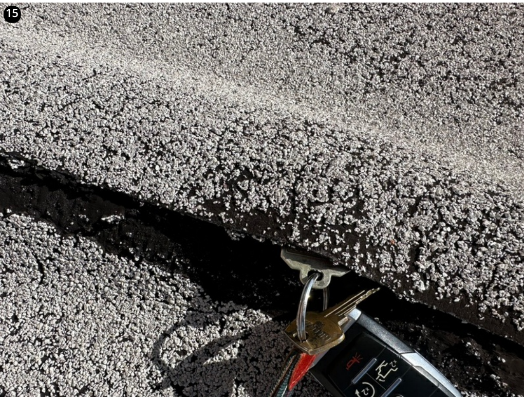
Open seam on a blister along--typical throughout.
